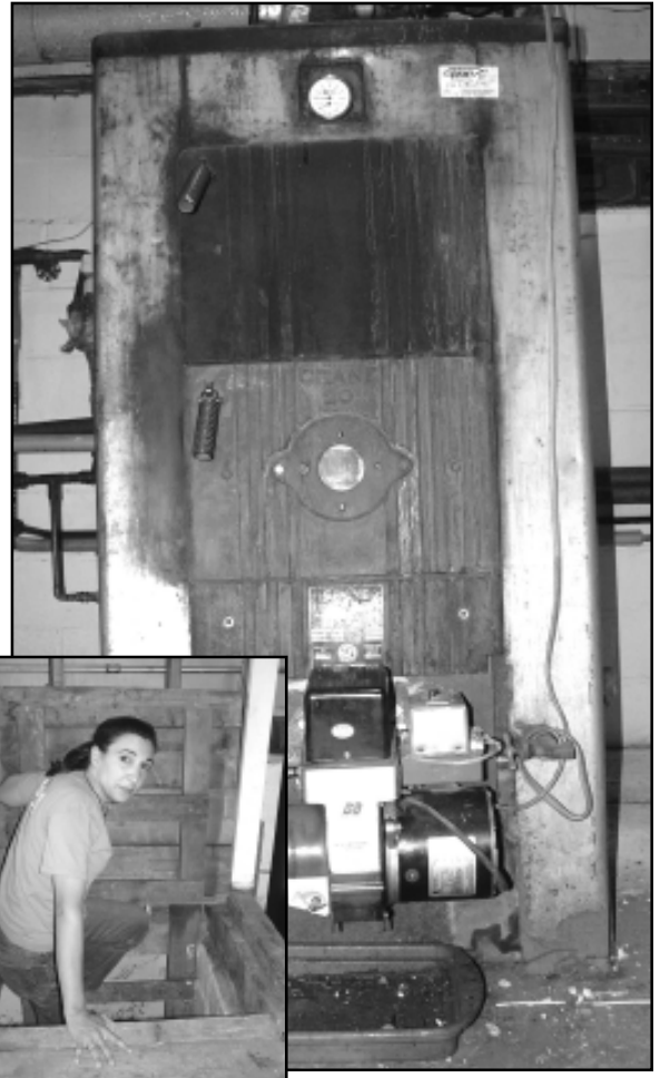
Top: Say goodbye to the Crane Model 20!; Inset: Your fearless Membership & Communications Director, none too happy about climbing down to the boiler.
